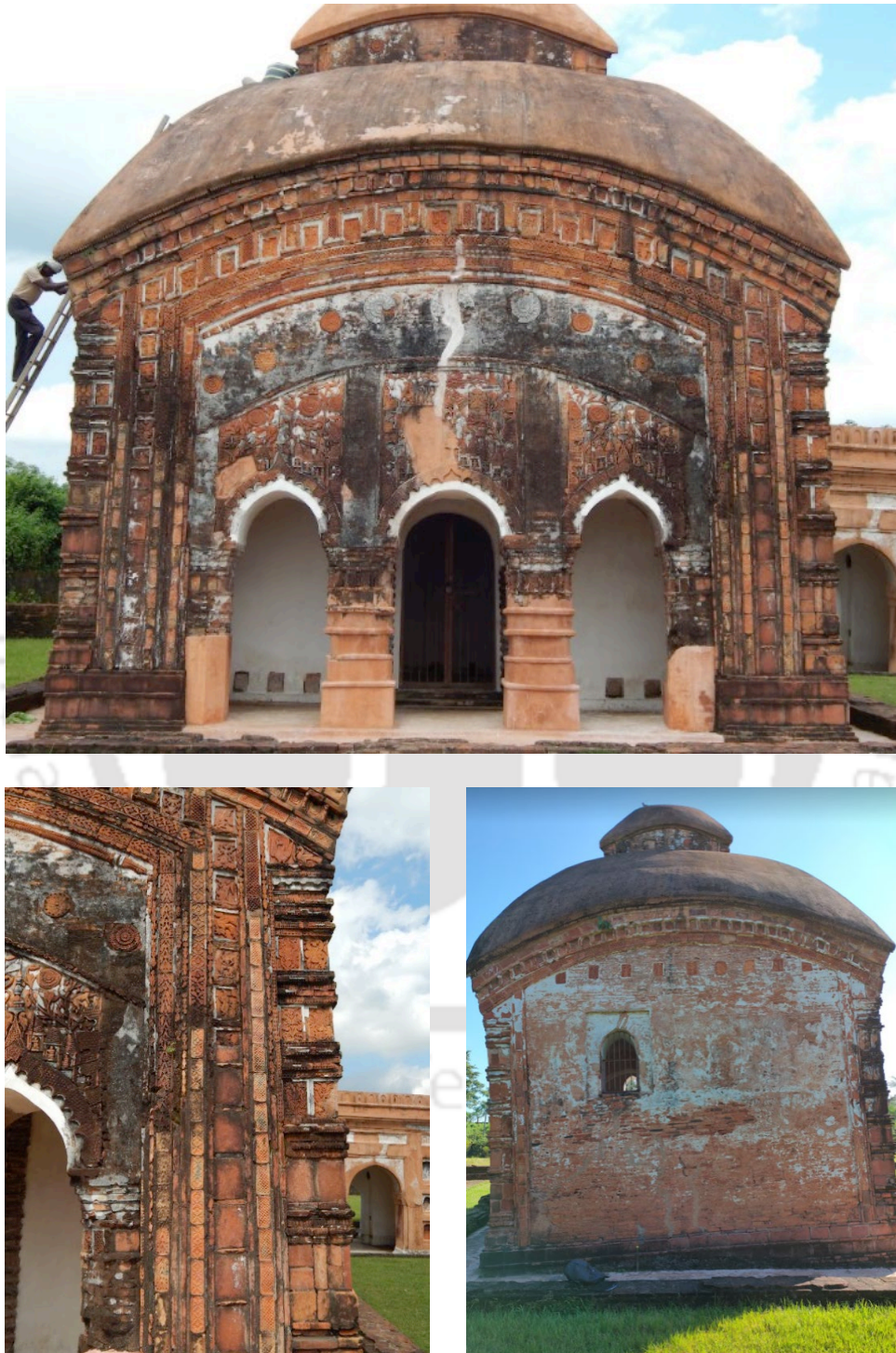
Appx A Fig. 1. 1 Ghanasyam House, Sivasagar- Photographs of various sections of the monuments
