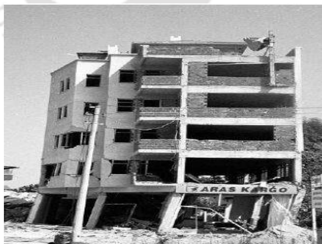
Figure 7.1: Damaged soft-story building subjected to Bhuj Earthquake, 2001
