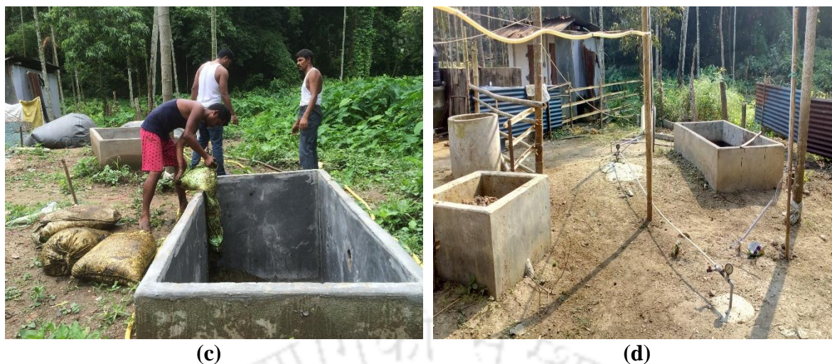
Figure 2.1. Installation of 4 m 3 biogas digesters at Aaoniati Satra near IIT Guwahati (a),(b) Deenbandhu type construction. (c) Feeding of cattle dung for inoculation. (d) Final setup of 4 m 3 biogas digesters.
