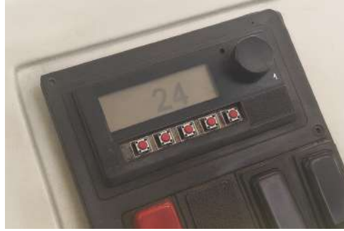
Figure 1.13: AC control panel (Source: Author's field study, 2023).
