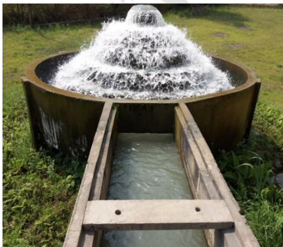
a) Main parshall flume
