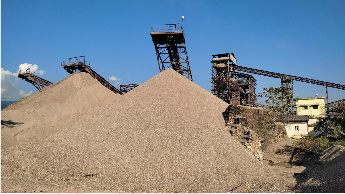
Figure 18: The central stone crusher that supplies gravel for the dam construction, located on the river island (Source: Author)
