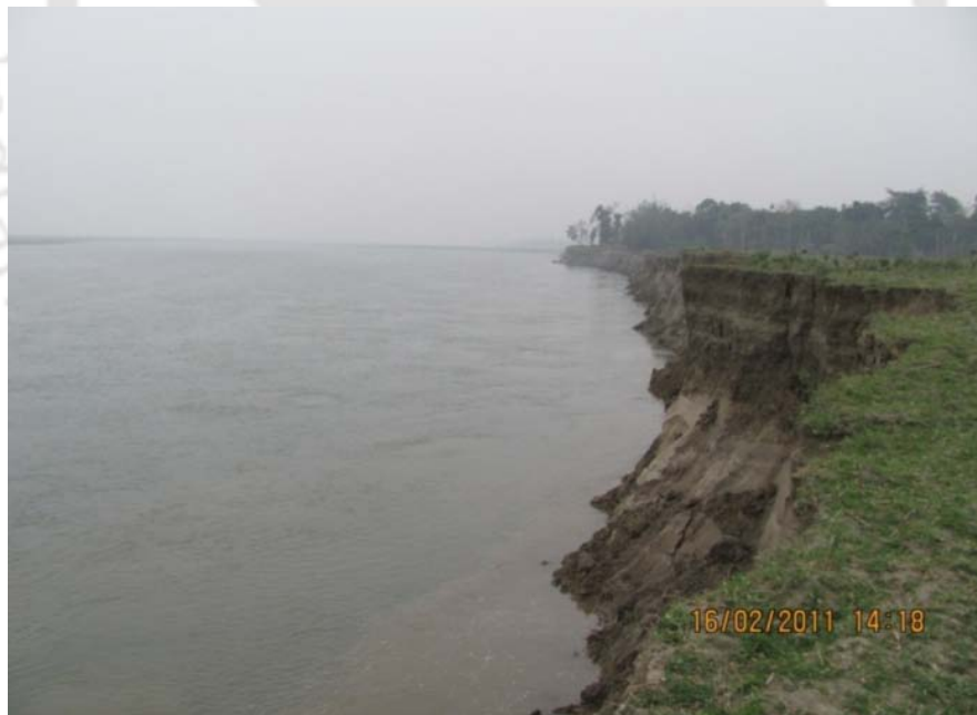
Figure 6.2 Bank facing erosion
