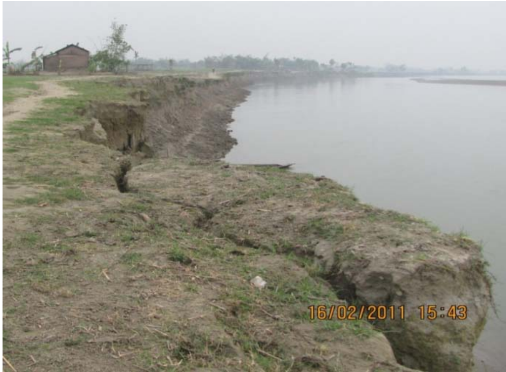
Figure 6.3 Bank on the verge of erosion
