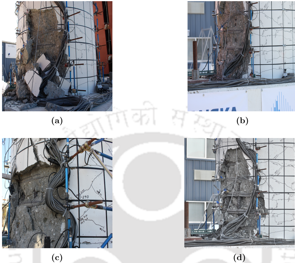
Figure 4.9: Damage during shake table test for different sequence; (a) EQ5, (b) EQ6, (c) EQ7, and (d) EQ8
