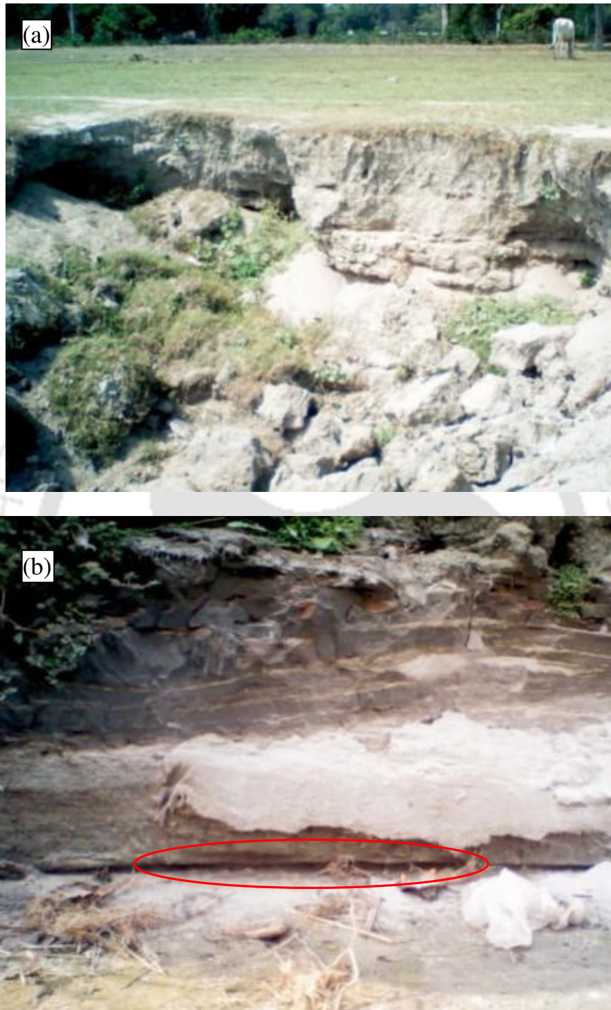
Fig. 3.3. Field photographs showing the seepage undercut and collapse along the Brahmaputra river bank: (a) collapse after seepage erosion (b) seepage undercut.
