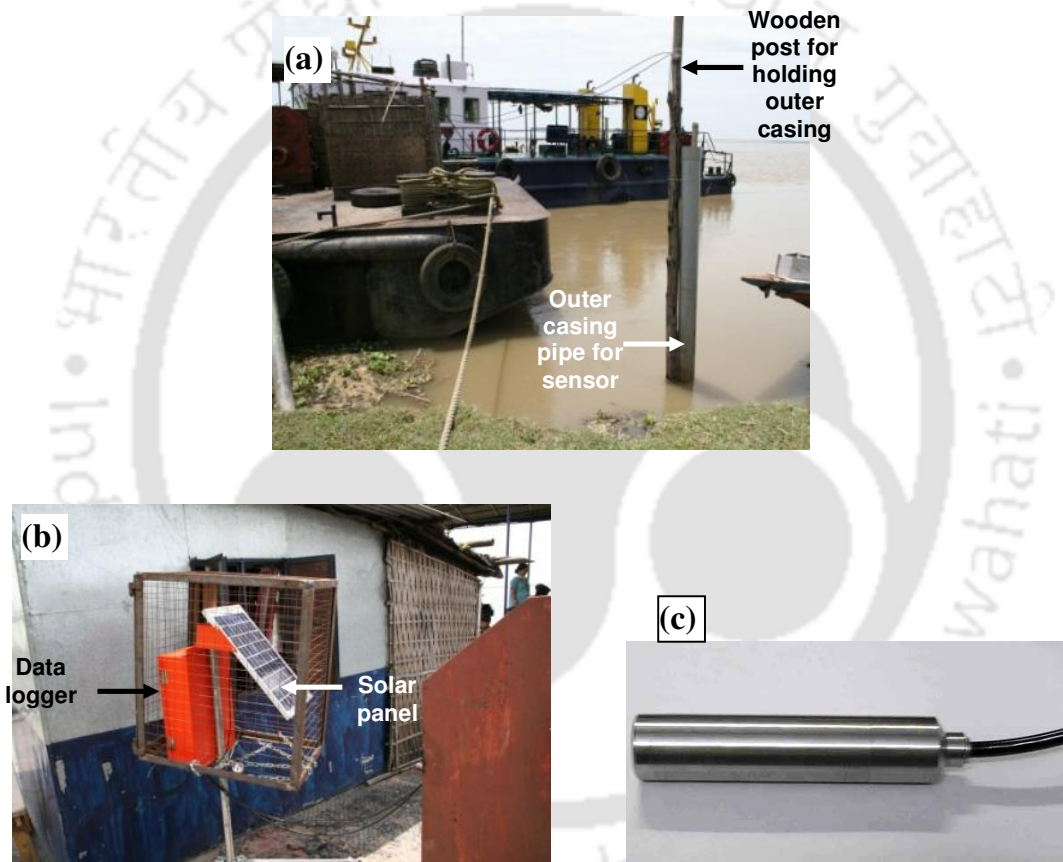
Fig. 3.13. In situ installation of the automatic stage recorder: (a) installation of pressor sensor inside the outer casing, (b) automatic data logger and the solar panel, (c) the pressor type sensor for stage recording.
