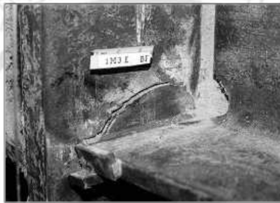
Fig. 2.1 Typical fracture paths at the welded beam-column connection [20]
