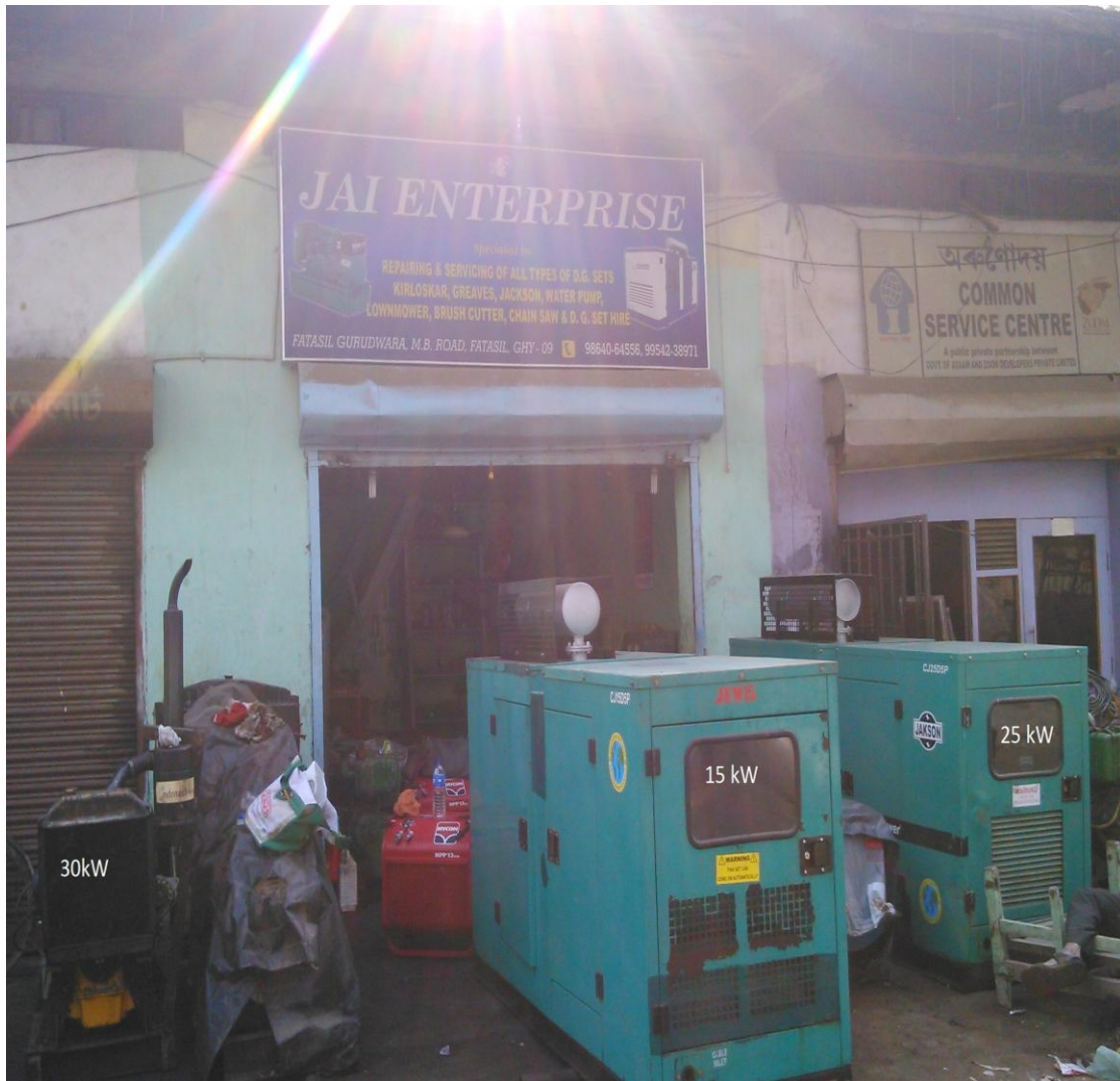
Figure 3.20 Three diesel generators used for field trial
