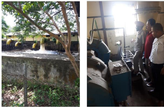
Ready to use pump system for Running of Model
