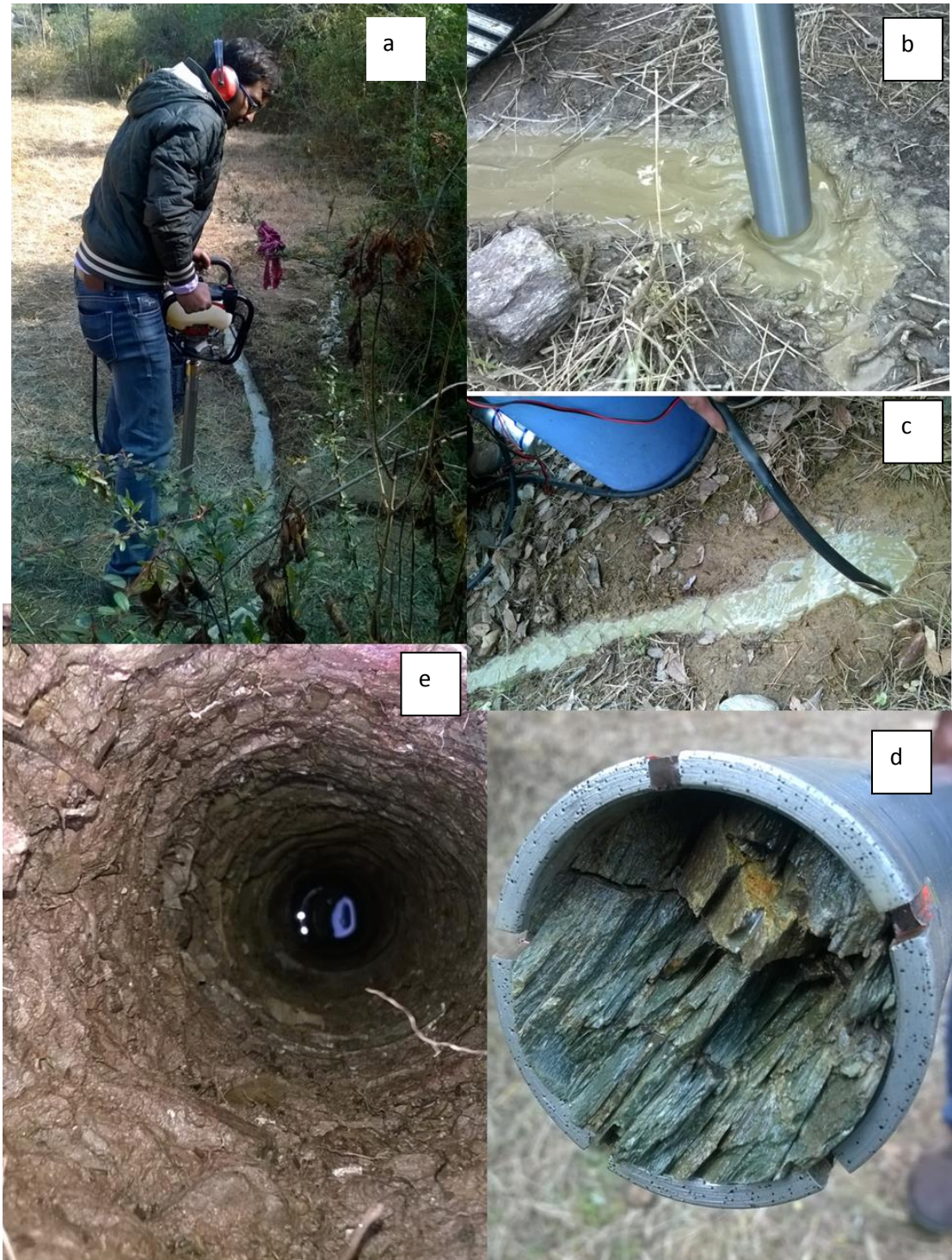
Photograph 5.1: Activities related to bedrock drilling for shallow borewell drilling using portable coring equipment (a), the slurry of drill fluid during drilling (b), well development by ejecting water through battery support pump (c), diamond bit with fracture core (d) and shallow borewell after borewell development (e).
