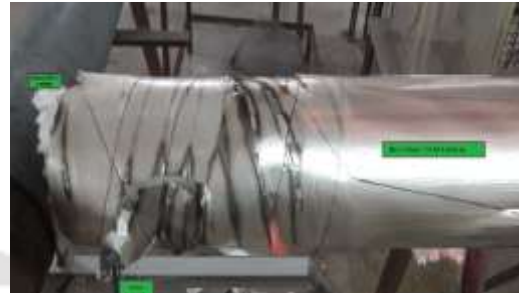
(b) Electric air heating chamber
