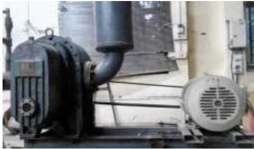
(a) Air blower
