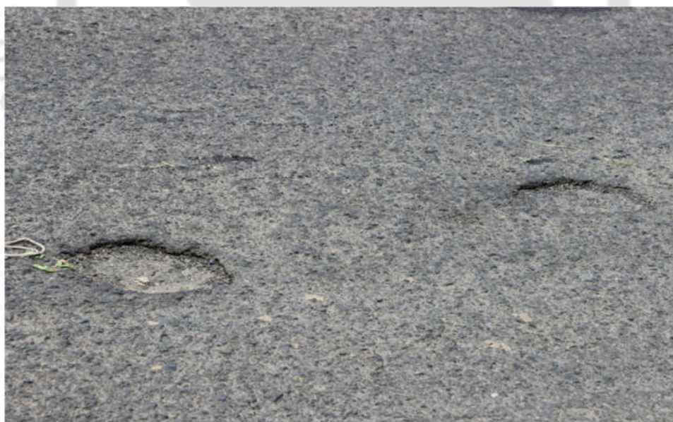
Photo 4.4 Potholes on pavement section NH-14GJ at Km. 381.00.
