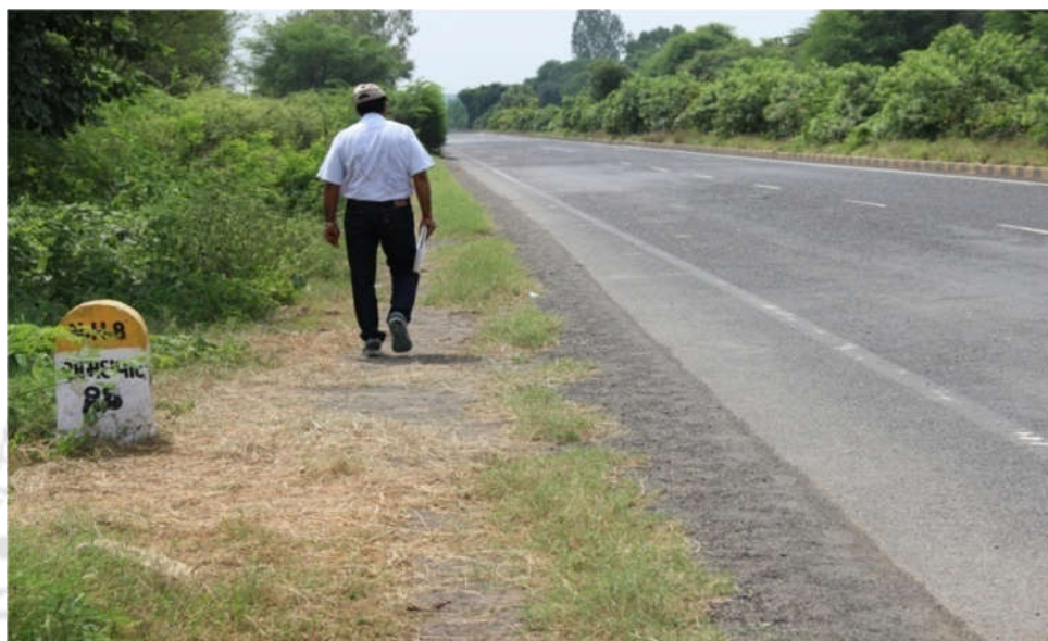
Photo 4.3 Ravelling on pavement section NH-8GJ at Km. 434.00
