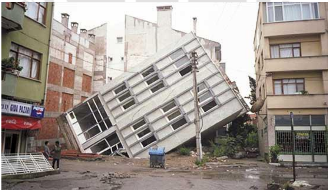
Fig. 1.1 Example of foundation failure due to seismic soil liquefaction in Adapazari region of Turkey during 1999 Kocaeli earthquake (after Sezen 2000)
