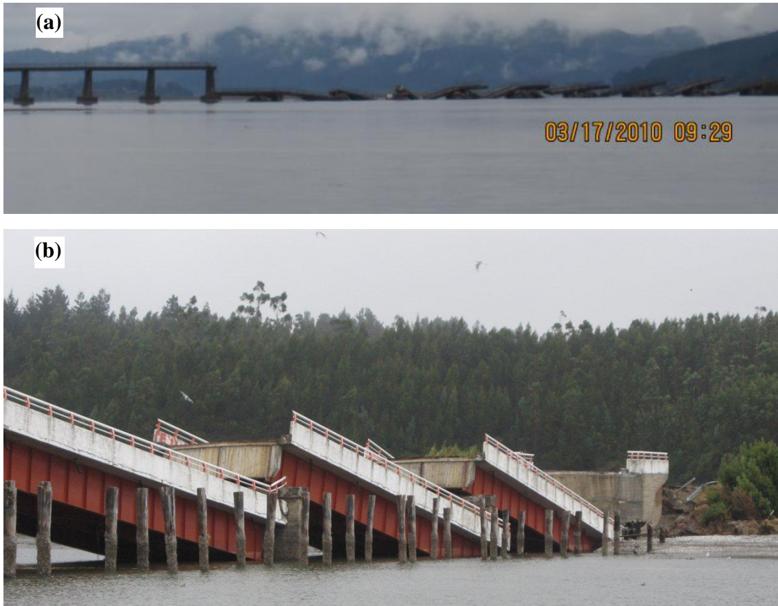
Fig. 1.2 (a) Elevation and (b) Sectional views of collapsed Tubul Bridge during Chile earthquake (after Yashinsky et al. 2010)
