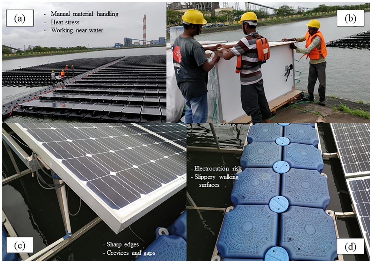
Figure 3.7. (a) A multitude of ergonomic hazards during installation; (b) work near water exposes the workers to a combination of hazards; (c) sharp edges and presence of electricity are occupational hazards, and (d) work on unstable floaters presents additional hazards (image: author)
