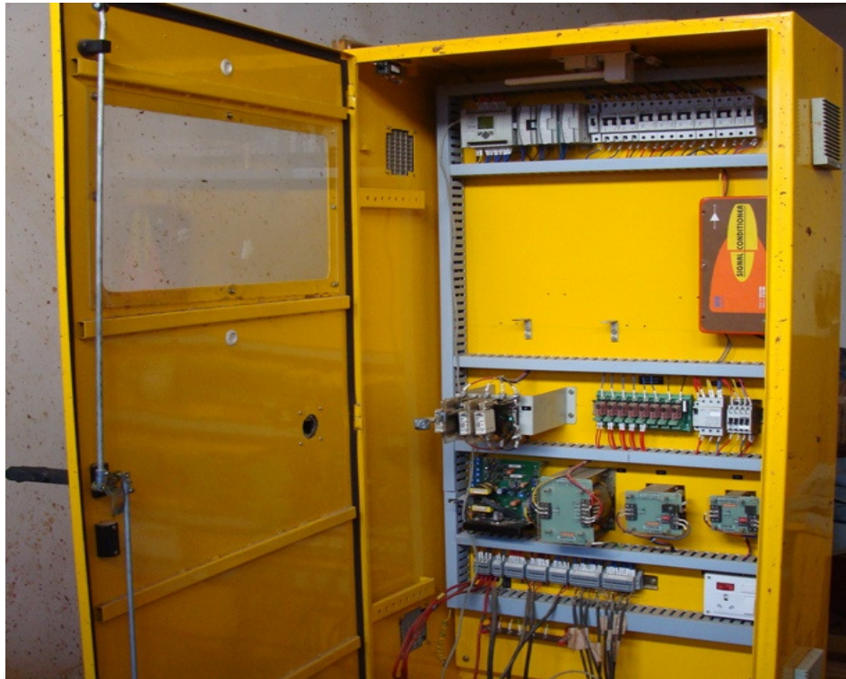
Fig.3.35: Close up view of the programme logic controller (PLC).
