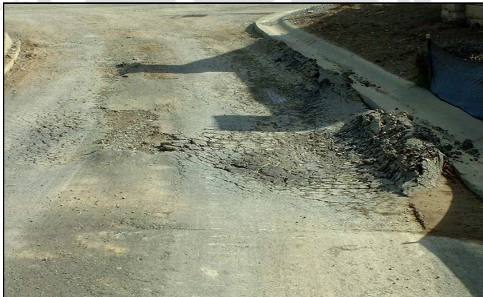
Photo 1.1 Pavement failure due to weak subgrade
