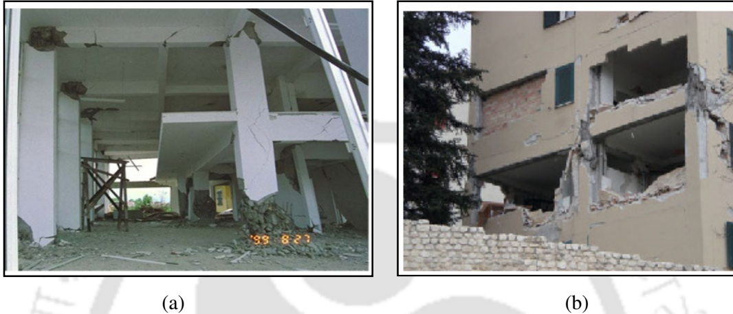
Fig.1.1 Distressed RC beam-column connections (a) during the 1999 Kocaeli, Turkey earthquake [Sezen et al. , 2000], (b) during 2009 L'Aquila Earthquake [Dr Anna Brignola, University of Genoa]
