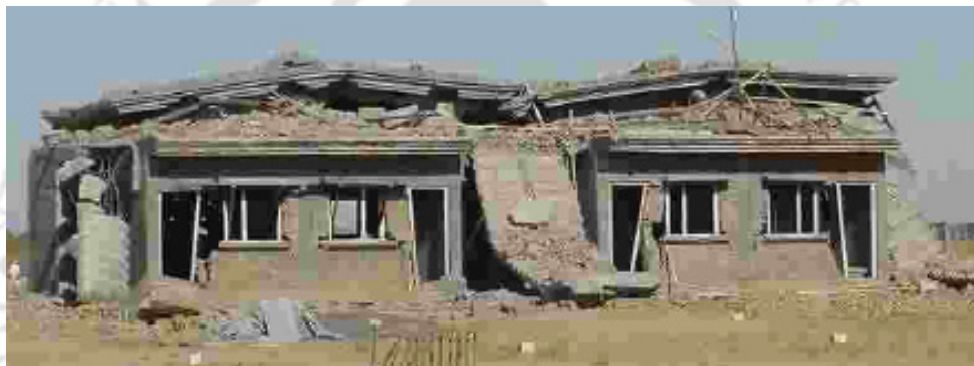
Figure 1.6. Collapse of the upper storey of a URM building under construction at Bhachau in Gujarat (Jain et al., 2001).
