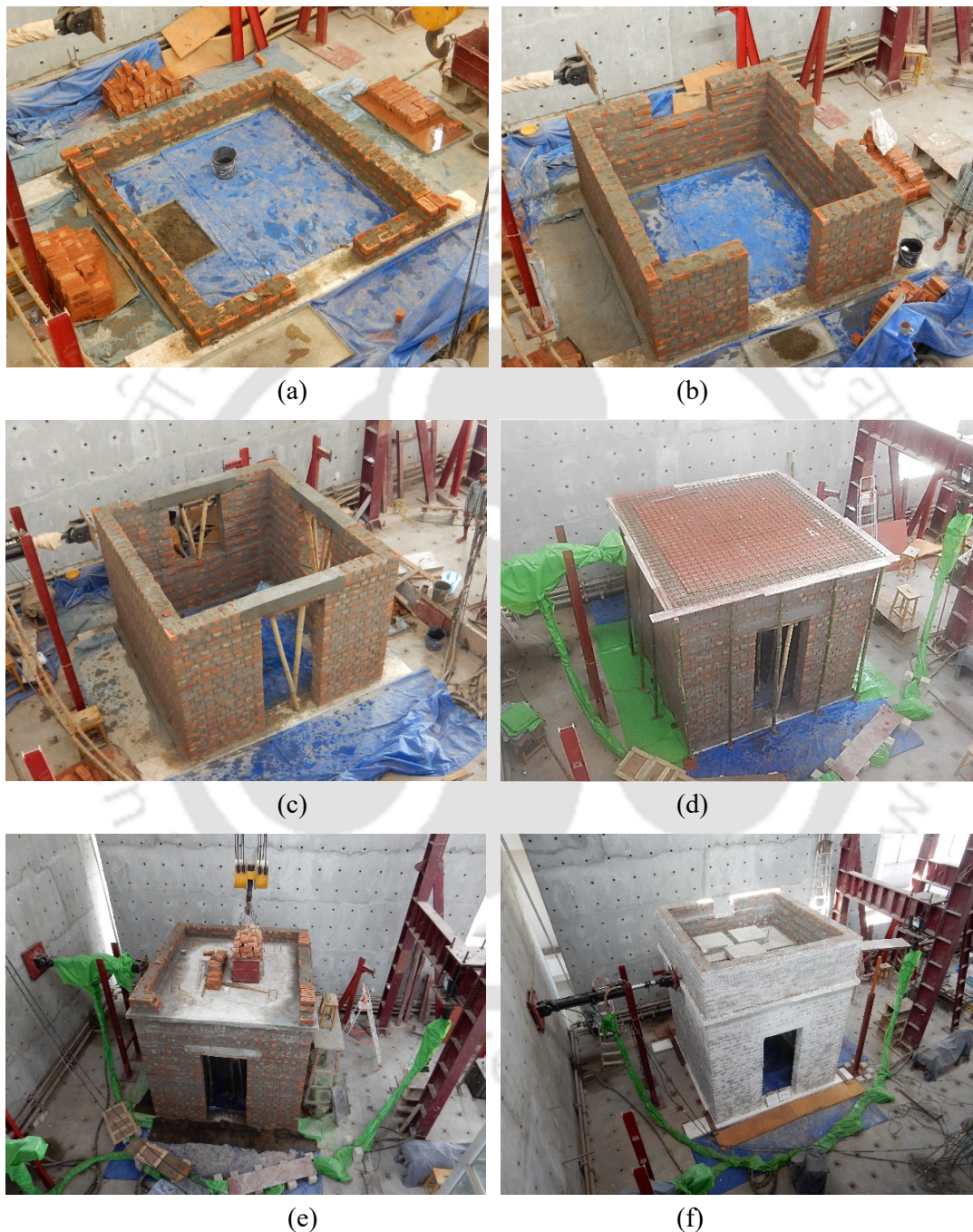
Figure 5.3. Stage wise construction of URM building up to: (a) base, (b) window, (c) lintel level, (d) roof level, (e) parapet wall, and (f) completion.
