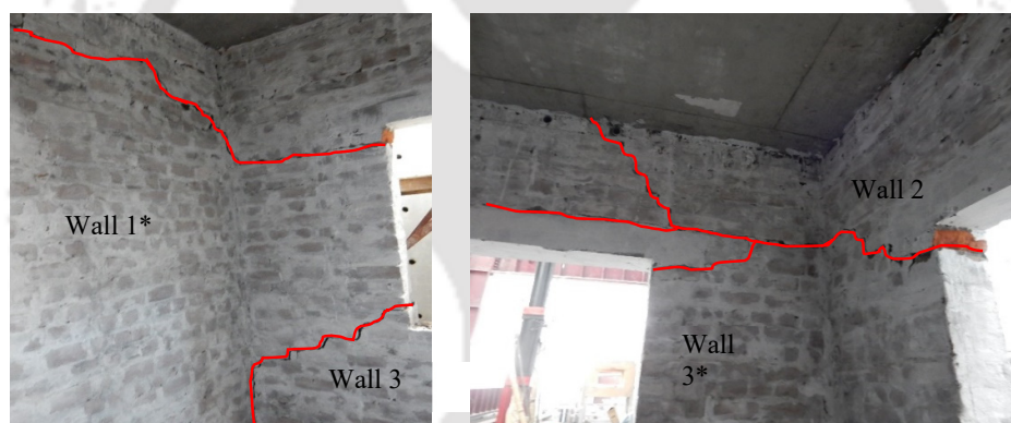
Figure 5.8. Damage observed in different walls inside the unstrengthened URM building during the lateral load testing.
