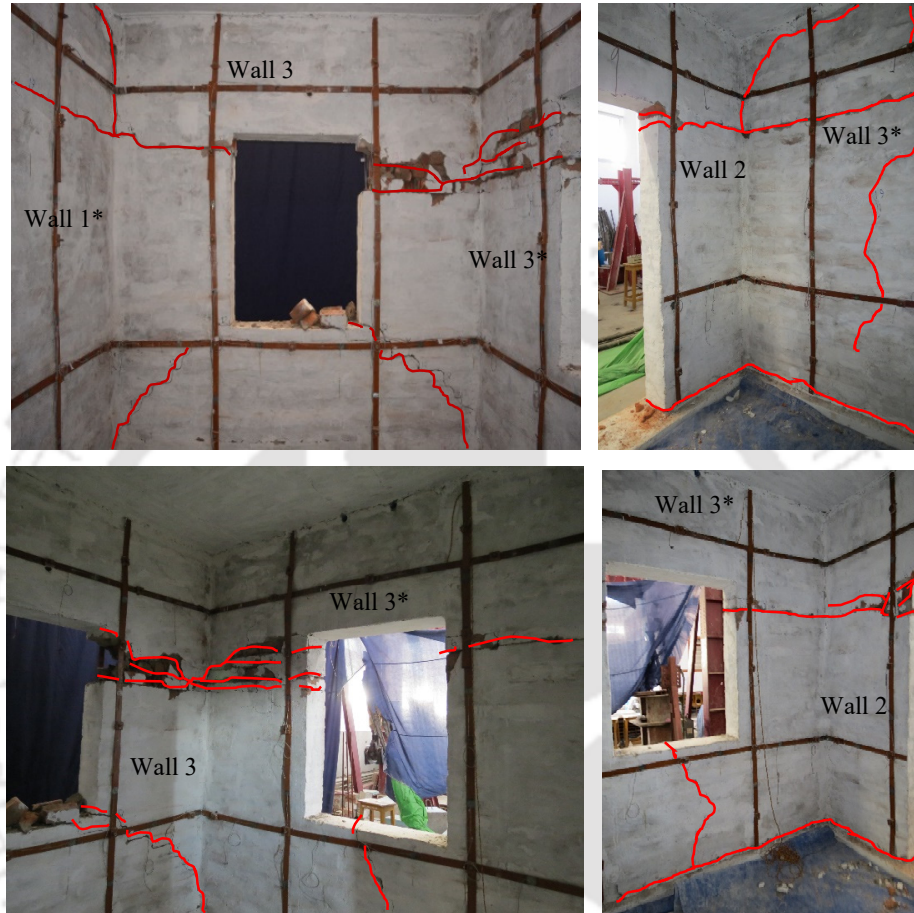
Figure 5.17. Damage observed in different walls inside the Model 2 during the lateral load testing.
