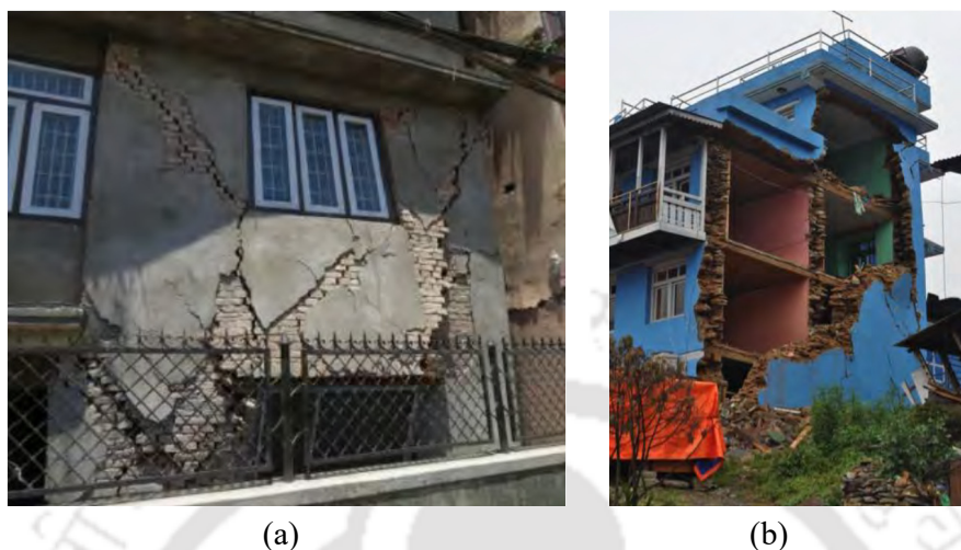
Figure 1.14. Performance of URM buildings during Nepal Earthquake: (a) in-plane wall damage, and (b) out-of-plane collapse of masonry walls (Lizundia et al. 2016).
