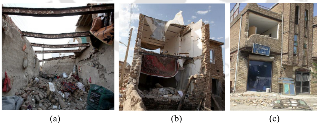
Figure 1.11. Performance of URM buildings during 2012 Iran earthquakes: (a) Failure of heavy steel jack-arch, concrete roofs and walls of URM buildings, (b) out-of-plane collapse of walls in URM buildings, and (c) buildings compliant with minimum code requirements survived the earthquake with minor damages (Razzaghi and Ashtiany, 2012).
