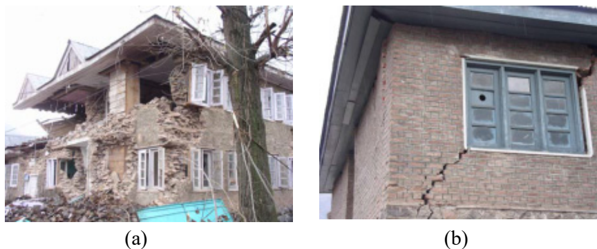
Figure 1.7. Failure in URM Buildings: (a) Out-of-Plane collapse of URM walls, and (b) Diagonal cracks in window openings and tilting of walls during North Kashmir Earthquake (National Disaster Management Division 2006).
