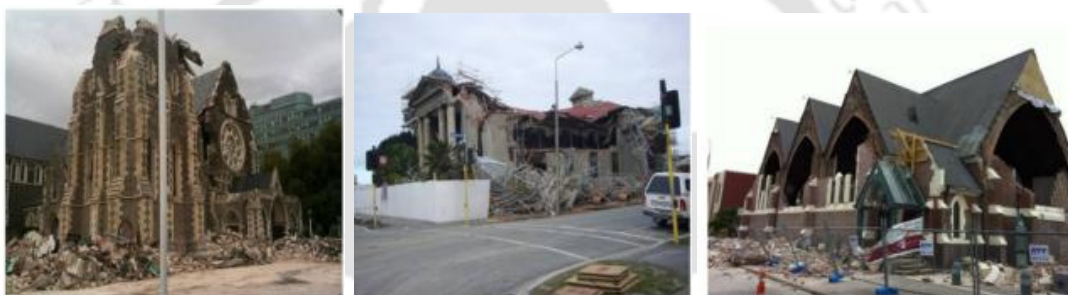
Figure 1.12. Severe Damage to several types of URM structures during the Canterbury earthquakes (Hare 2013).
