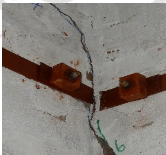
Figure 5.13. Steel band failure at the junction of Walls 2 and 3*.
