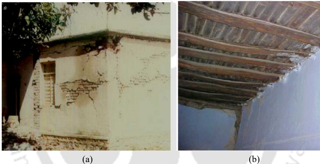
Figure 1.4. Type of URM buildings: (a) Overview of unreinforced brick masonry with timber roof, (b) Structural details of roof (Jain, 1993).
