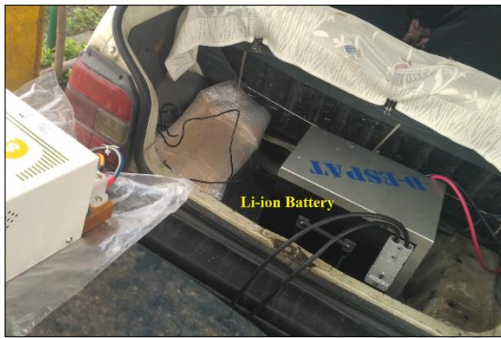
Figure 3.4: Li-ion battery installation,
