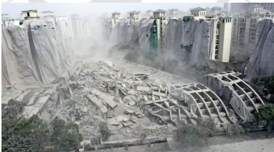
(e) Debris of residential towers few minutes after demolition by controlled explosion
