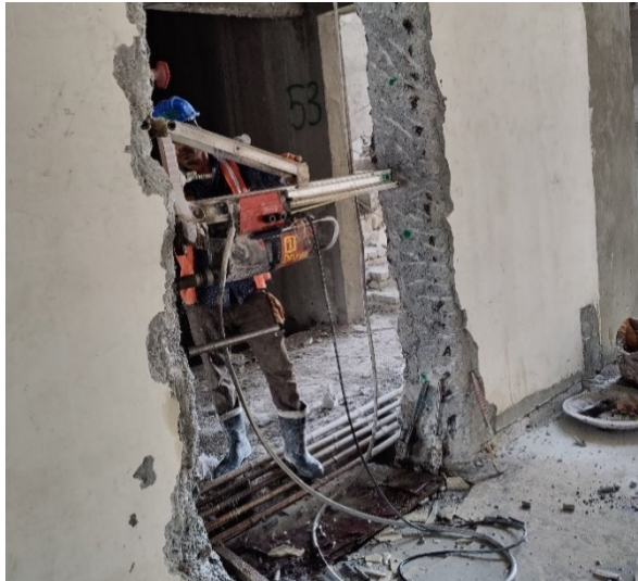
(a) Drilling of bore holes in shear walls using diamond core cutting machine
