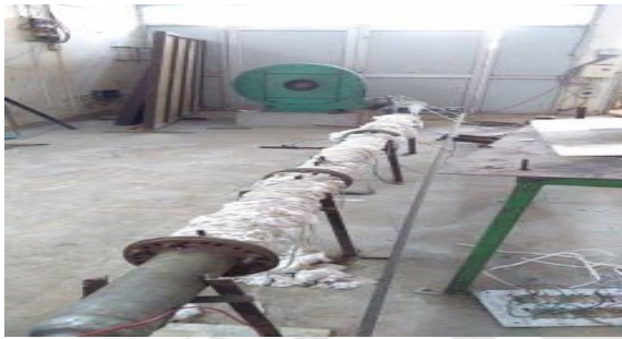
Pipeline connection with blower
