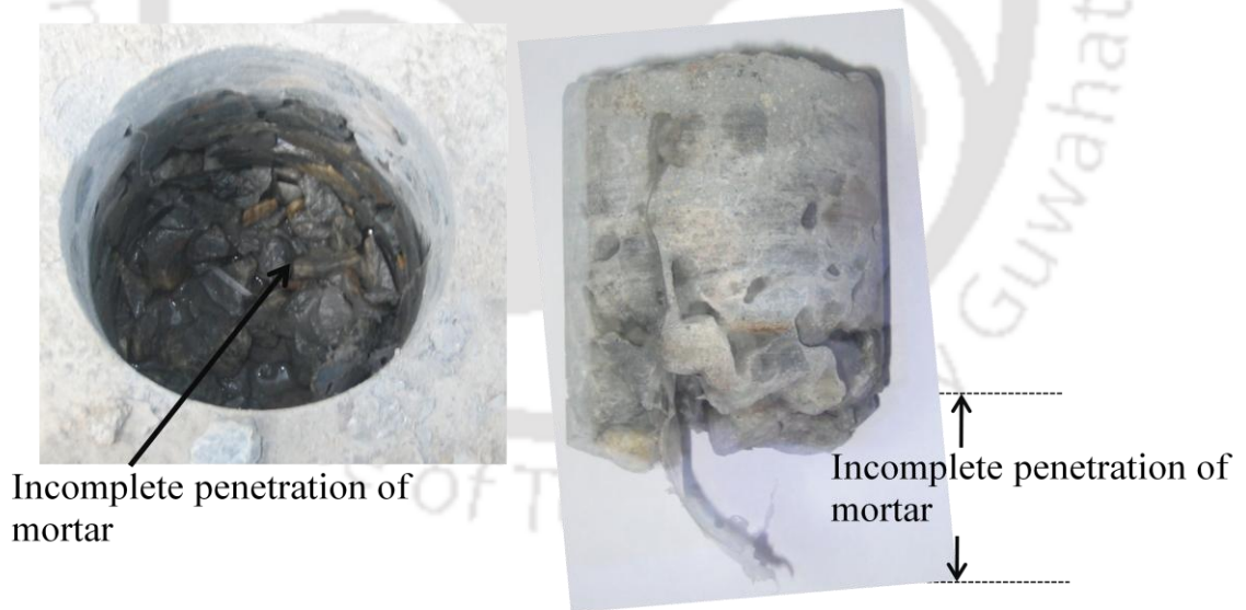
Figure 3.4: Incomplete penetration of mortar in grouting method.
