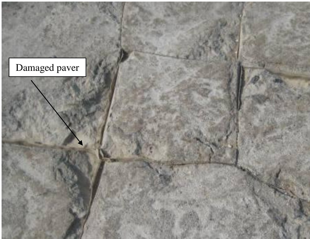
Figure 4.7: Damaged pavers observed in 120 mm thick PCCBP test section.
