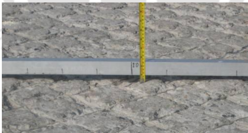
Figure 4.4: Rutting in 50 mm PCCBP test section.
