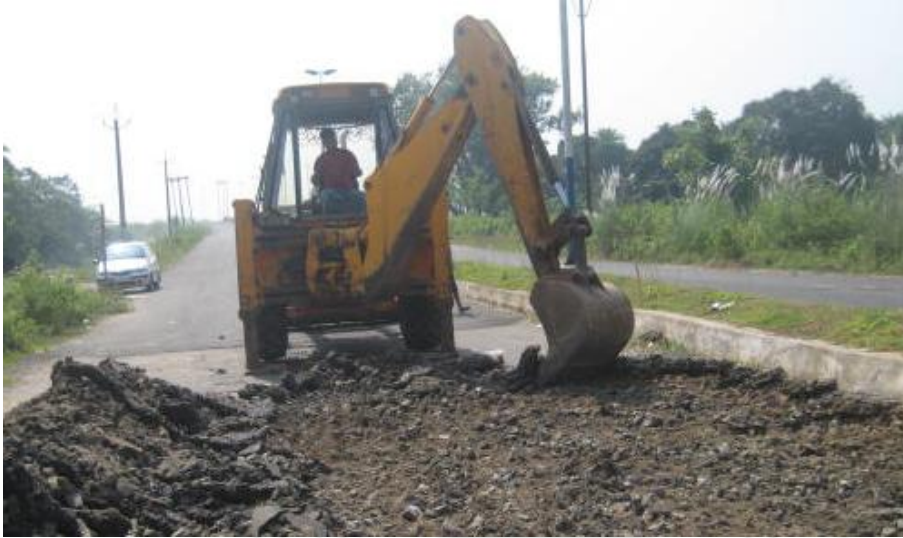
Figure 3.7: Excavation and removal of the top layers of the existing bituminous pavement.
