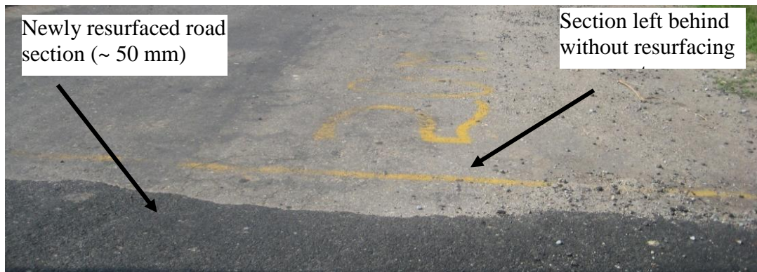
Figure 3.11: A section of the road left behind while resurfacing the road stretch on which the test pavement was constructed.
