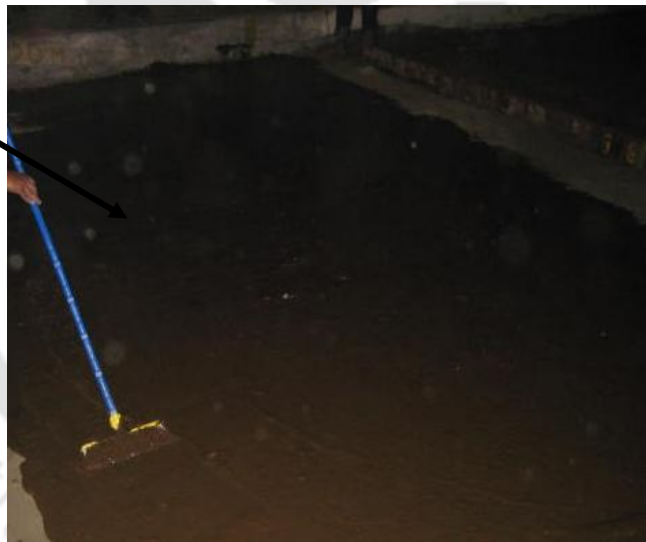
Figure 3.12: Application of adhesive prime coat Gellix over existing bituminous pavement, after surface preparation.
