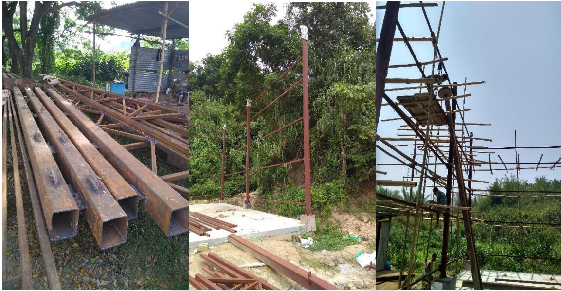
Figure 10.15 Photographs of steel sections for columns & beams (left); erected column sections (middle); and casting of columns & beams (right)
