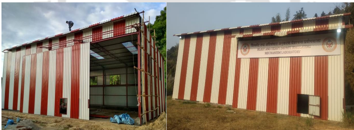
Figure 10.18 Blast Resistant Framed structure used as Blast and Heavy Impact Simulating Mechanism (BHISM) Laboratory, IIT Guwahati
