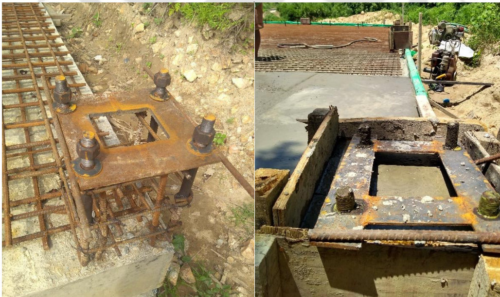
Figure 10.14 Photographs of laying (left) and casting (right) of column base with Base plate
