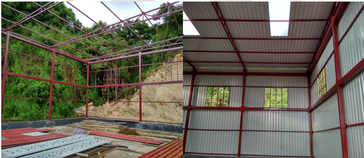
Figure 10.16 Photographs of the framed structure before (left) and after providing walls with CGI sheets (right)
