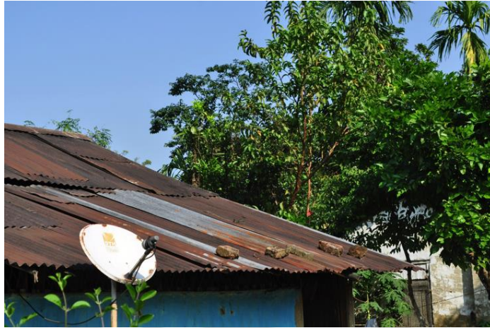
Figure 44. A rural house with DTH connection in Belkona
