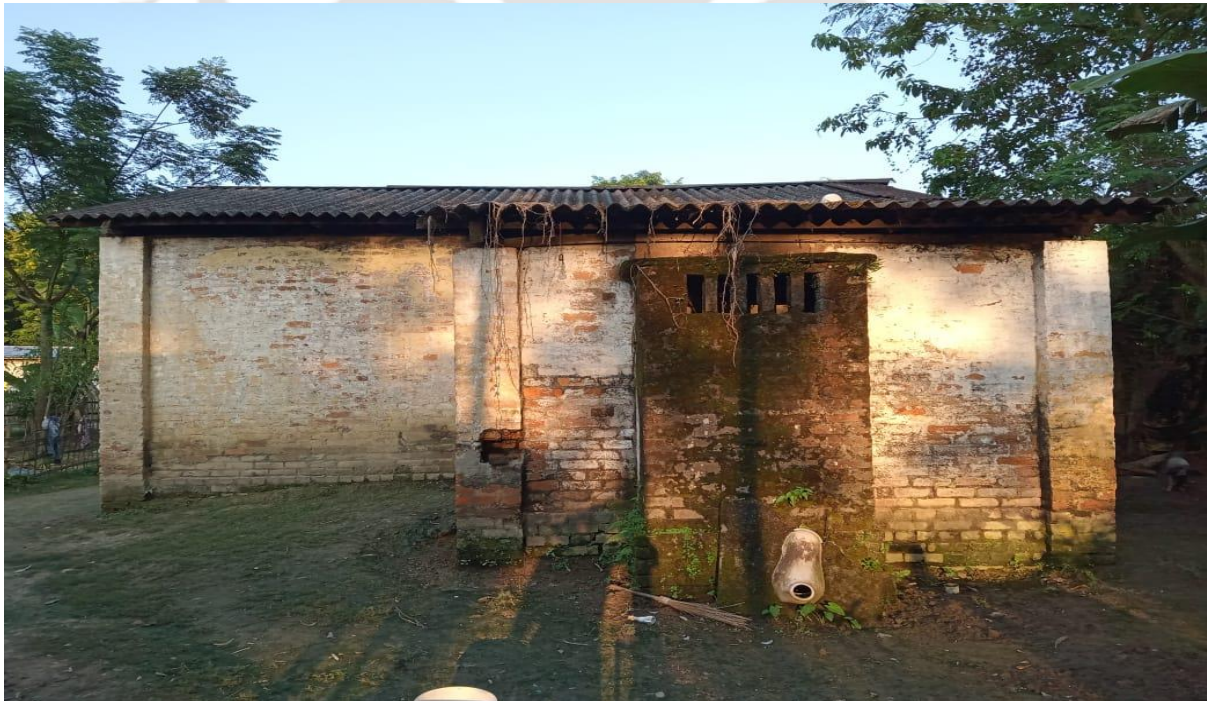
Picture 4.5: A toilet in workers' quarter
