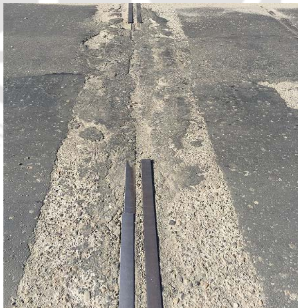
Fig. 1.6 Damage to the expansion deck joint in a conventional bridge type.
