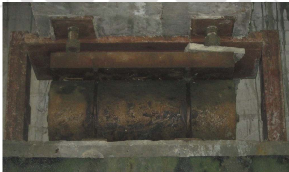
Fig. 1.5 Rusting of bearing joint in conventional bridge type
