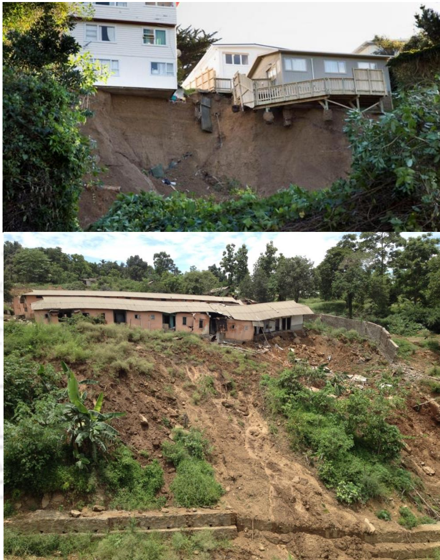
Figure 1.1 Examples of rainfall induced slope failures
