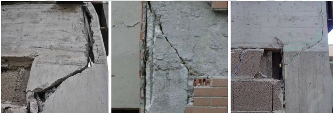
Fig. 1.1. Local shear failure of columns due to infill-frame interaction (Cavaleri and Di Trapani 2015).
