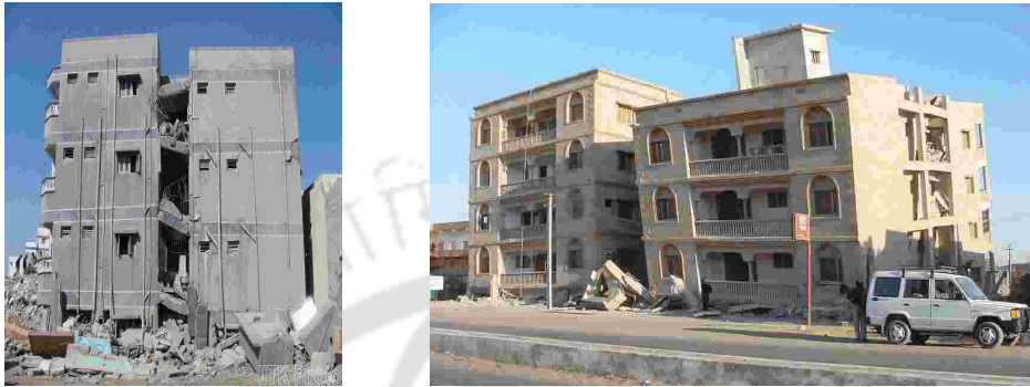
Figure 1.1 Collapse of open ground storey RC frame residential buildings with small to large openings at Bhuj during 2001 Bhuj earthquake [Source: www.nicee.org accessed on 05 February 2018].
