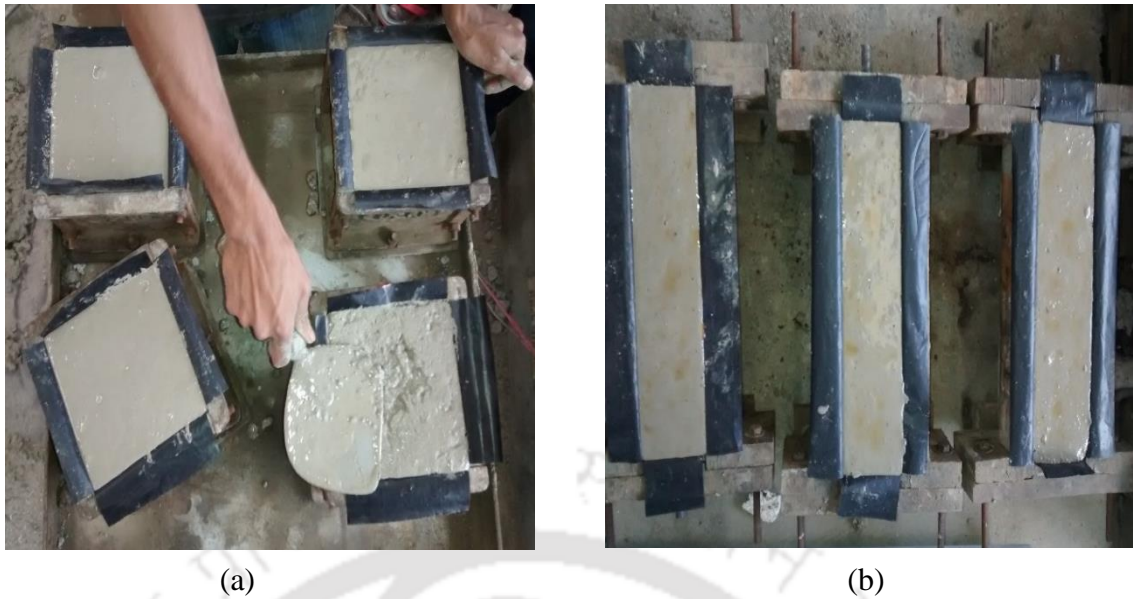
Fig. 3.5: Compaction of geopolymer concrete for (a) Cube specimens (b) Prismatic reinforced specimens
