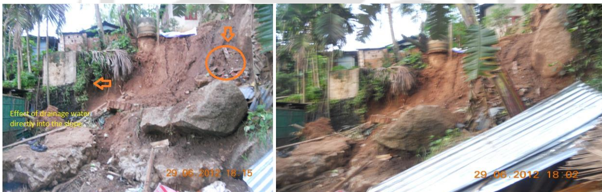
Figure 3.4 Landslide at Mathuranagar, Santipur, Fatasil hill ( 26^{\circ} 09' 50.5'' N, 91^{\circ} 43' 41.7'' E) (Goswami, 2013)
