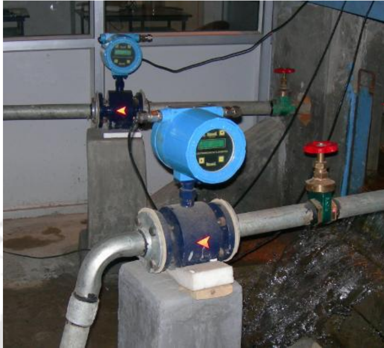
Figure 2.6 Electromagnetic flow meters for measuring seepage discharge
