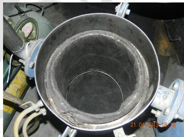
Fig. 4 Tar deposited in fine filter
