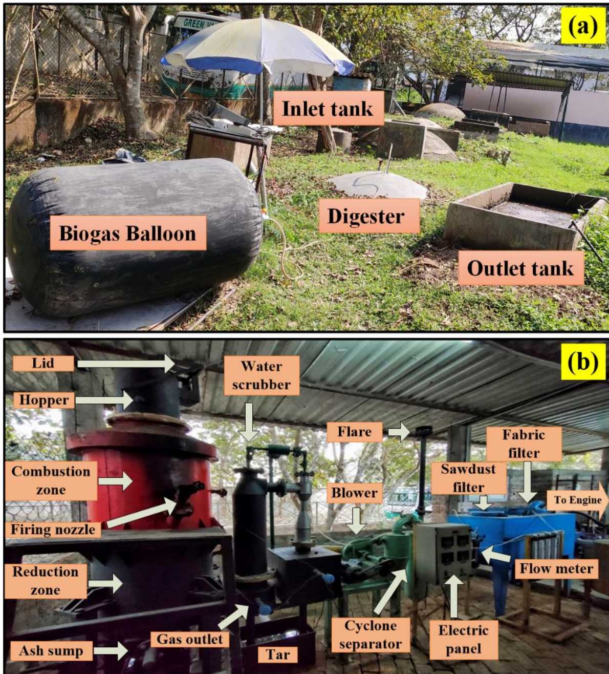
Fig. 3.5 Photograph of gaseous fuel generation units (a) anaerobic digester and (b) downdraft biomass gasifier
