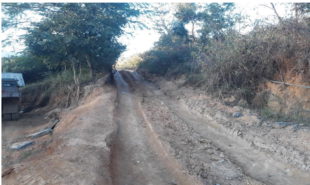
Plate 11: Pitiable condition of the road in Teiseng village (Photo: Author)
