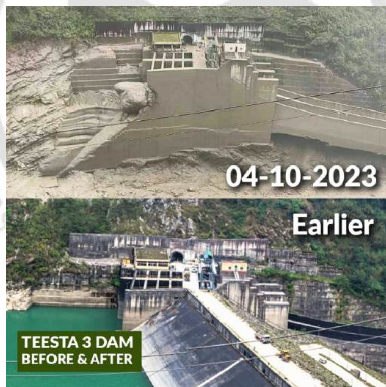
Figure 1.1: Pre and Post GLOF condition of Teesta 3 Dam as indicated by before and after flood image (Source: SANDRP (2023)).
