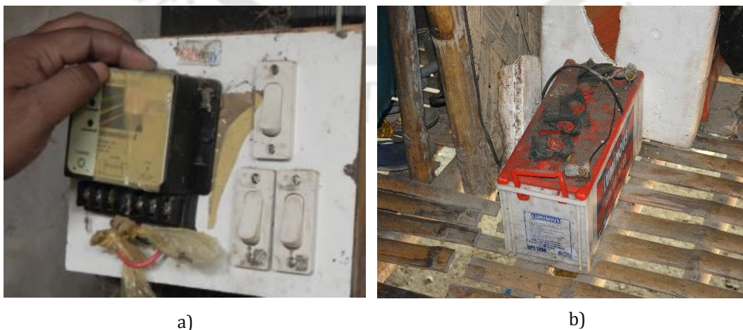
Fig. 2.4 Component faults as observed during study (a) Bypassing of charge controller (b) Damaged battery due to direct charging
