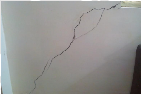
(f) Cracks in the wall.
