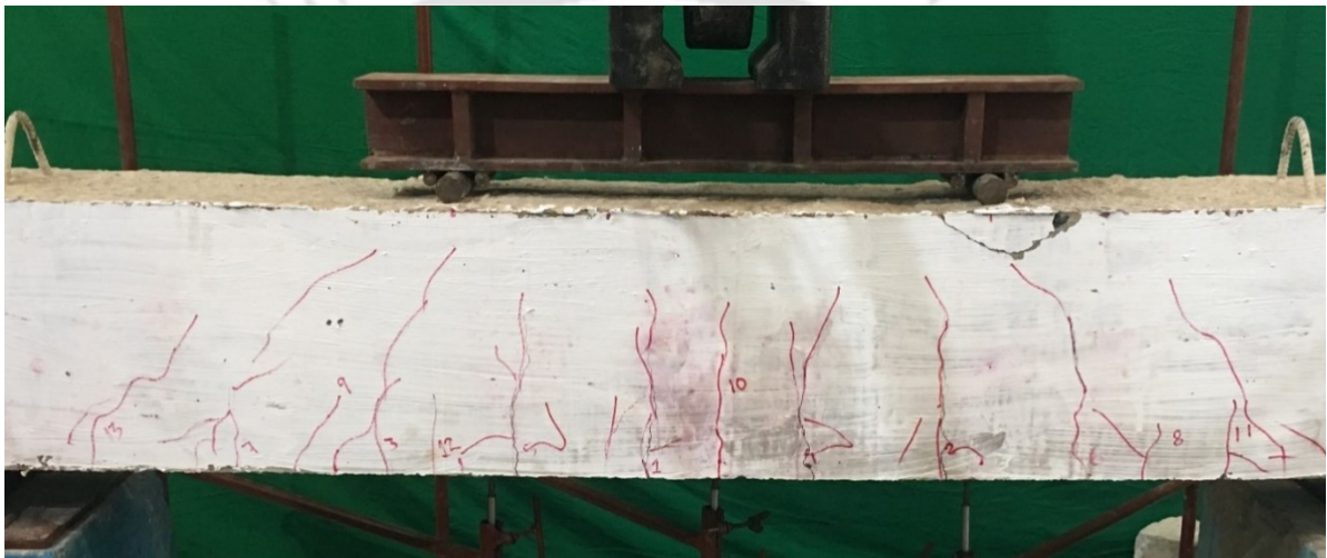
Figure 6.10 (b): Cracks in PCC jacketed RC beam, B9J.
