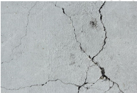
(c) Shrinkage cracks in concrete.
