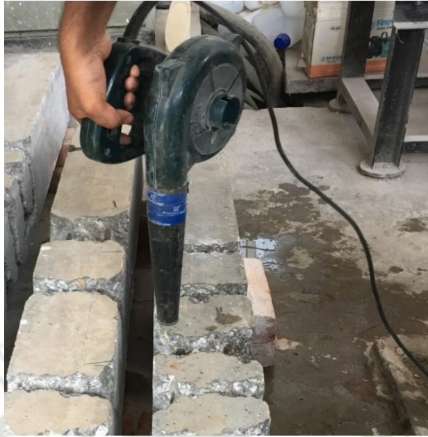
Figure 5.9: Use of air blower for removal of dust particles from inside the cracks.
