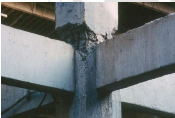
(e) Cracks in beam-column joint.
