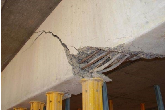
(a) Failure due to overloading in beam.
