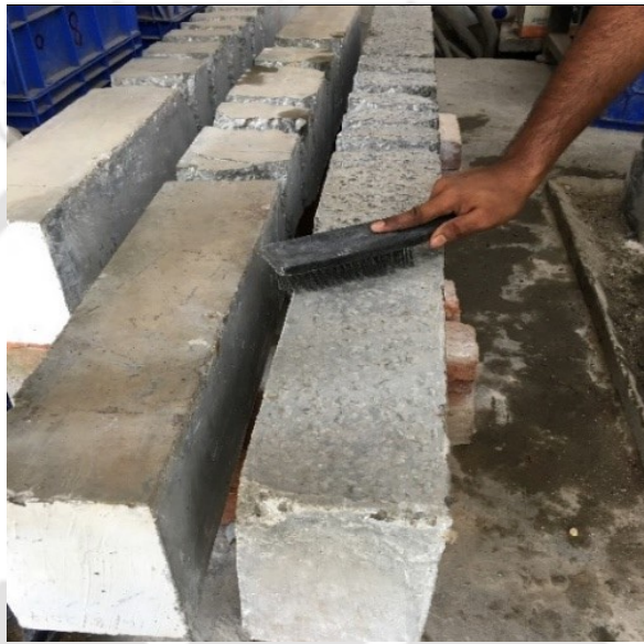
Figure 6.4 (a): Removal of the loose particles from the surface by iron brushing.
