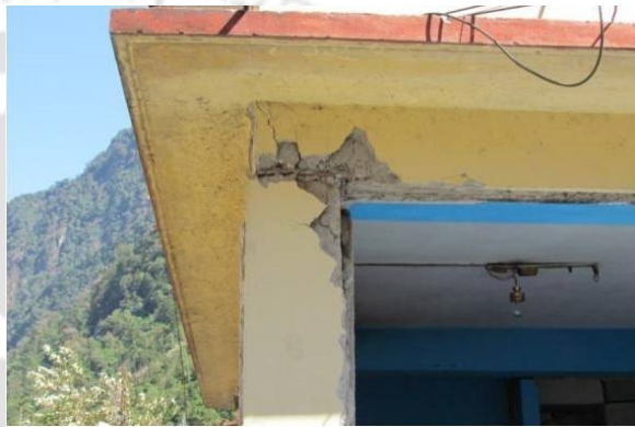
(d) Cracks in beam-column joint due to earthquake.
