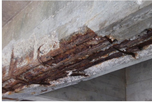
(b) Failure due to corrosion in beam.
