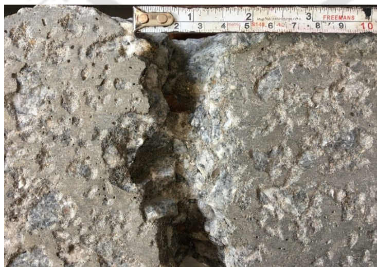
Figure 5.8: Crack width in the damaged RC beam after enlargement for repairing.
