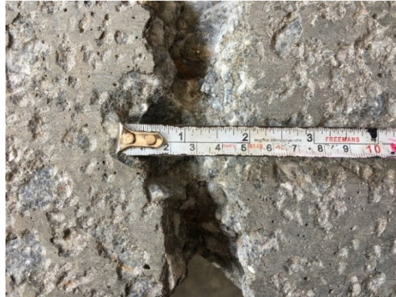
Figure 6.4 (c): Crack ready for being repaired.
