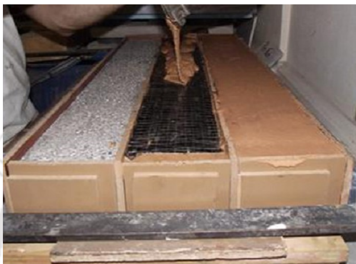
Figure 1.22: Placing CFRP sheet and geopolymeric on the concrete surface ( Vasconcelos et al. [51]).
