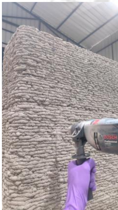
Step 10. Drilling in the wall (at desired location as shown in Fig. 7b)
