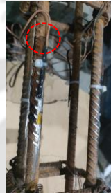
Step 7. Rest for 30 minutes, then applying 2 nd layer of epoxy till wire rapping
