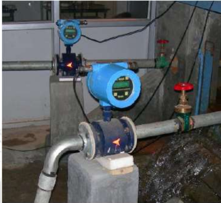
Figure 2.6 Electromagnetic flow meters for measuring seepage discharge
