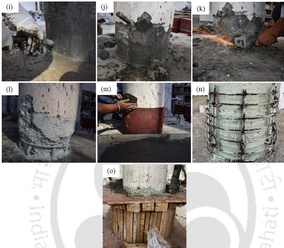
Fig. 5.5. Rehabilitation methodology (a) drilling of holes to facilitate epoxy injection; (b) chiseling of loose damaged concrete; (c) cleaning of drilled holes and concrete surface using air blower; (d) placing of aluminium nozzles into drilled holes; (e) bringing the inclined pier to vertical position using chain-pulley system; (f) application of acrylic modifier over the concrete surface; (g) application of polymer mortar; (h) epoxy injection pump; (i) epoxy grouting; (j) sealing of nozzles; (k) cutting of nozzles after curing of epoxy; (l) application of bonding agent after chiseling of polymer mortar and cleaning of concrete surface ; (m) casting of concrete; (n) application of bonding agent after hacking of concrete surface and installation of reinforcement cage application of bonding agent; (o) casting of concrete jacket.
