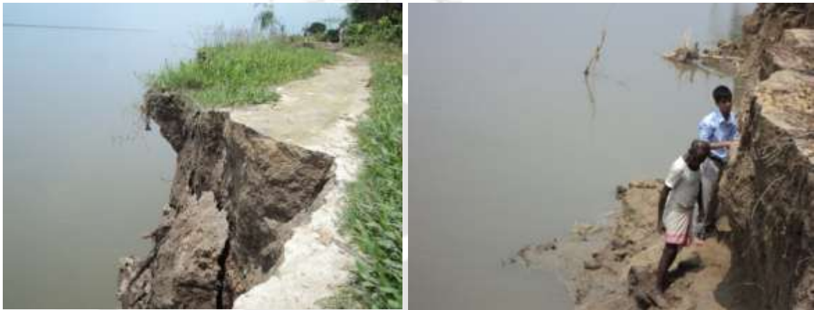
Figure 3.11 Erosion sites of Gamerighat
