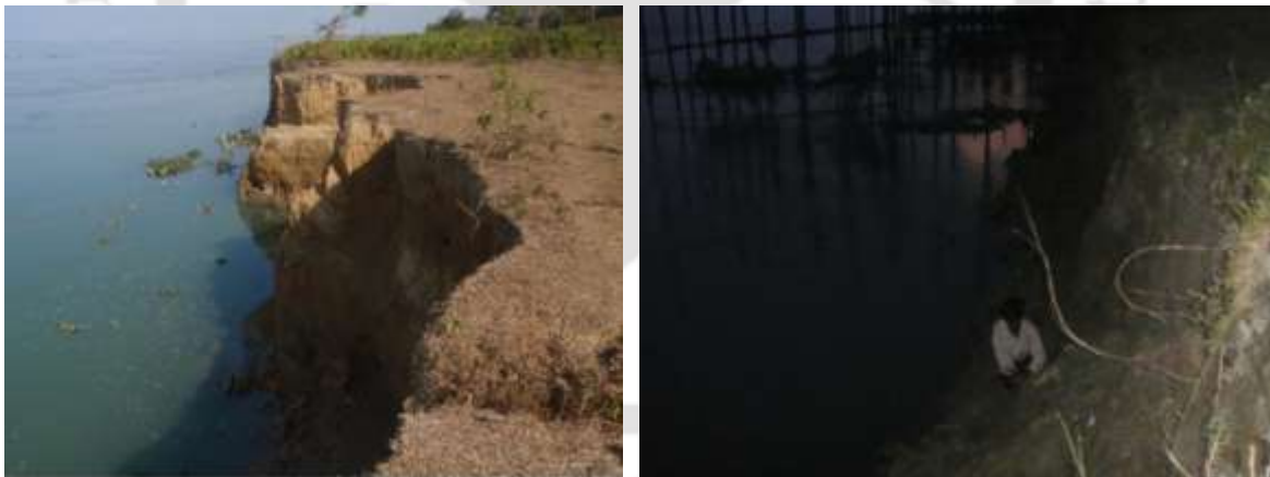
Figure 3.7 Erosion sites of Rohmor
