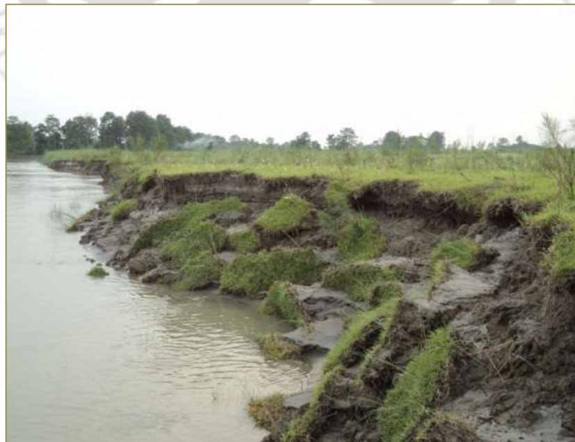
Figure 6.8 Bank failure of a composite bank in erosion site D
