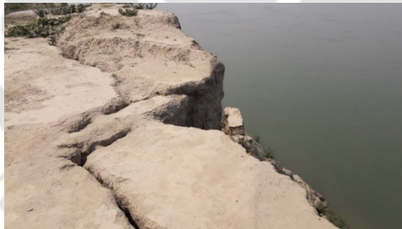
Figure 2.13 An earthen embankment with a large crack, Morigaon, Assam, India
