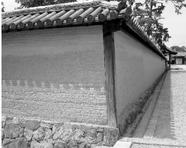
Fig. 2.3. Rammed earth walls surrounding Horyuji Temple, Japan (constructed ~1300 years ago) (Source: Henman, 2004).
