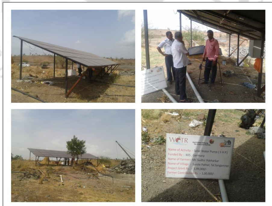
Figure 4.13 Top left -Solar PV powered water pumping system in Sarole Pathar Village. Top right- Discussion with the farmer (owner of the system) to get the system's information. Bottom left-system with water well. Bottom right - system specifications.
