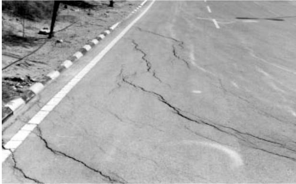
Fig. 1.2 Damage in pavement founded on expansive soil.
