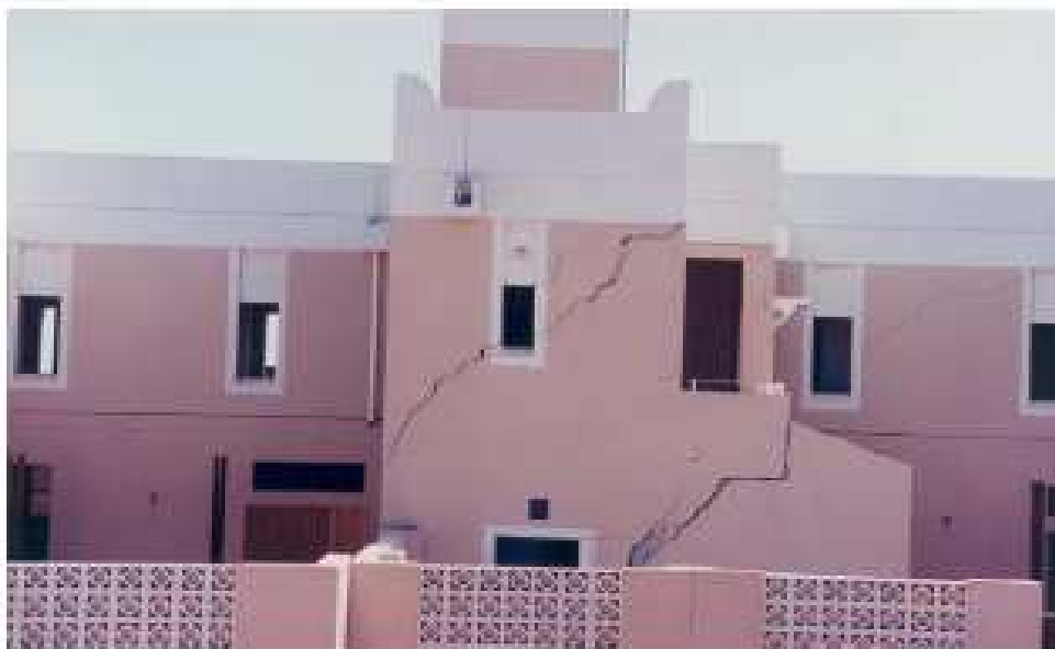
Fig. 1.1 Structural damage due to ground heave (Al-Rawas et al. 2005)
