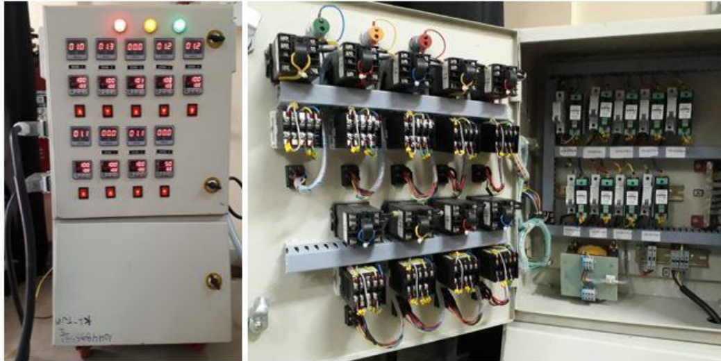
Figure A2-29 Temperature Control box
